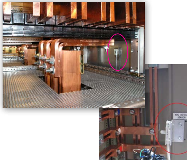
Figure 4. Examples of Arc-Flash relay light sensors installation in switchgear.
